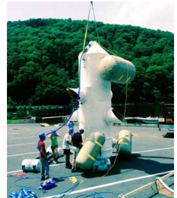
Pontoons were attached to the Systems to allow them to be floated and towed to installation points off Arrowpoint.
