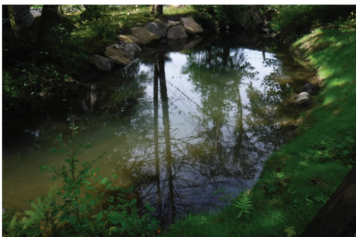
Completed sediment trap clean out at the intersection of Hawes Brook and North Shore Road.
